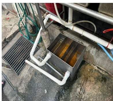
Fig. 2: The improper grease trap installation
