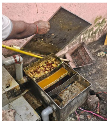
Fig. 3: The grease trap is not well maintained
